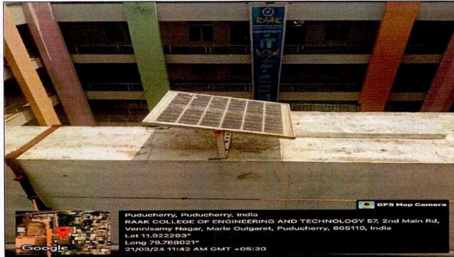
SOLAR PANELS ON THE ROOF TOP
