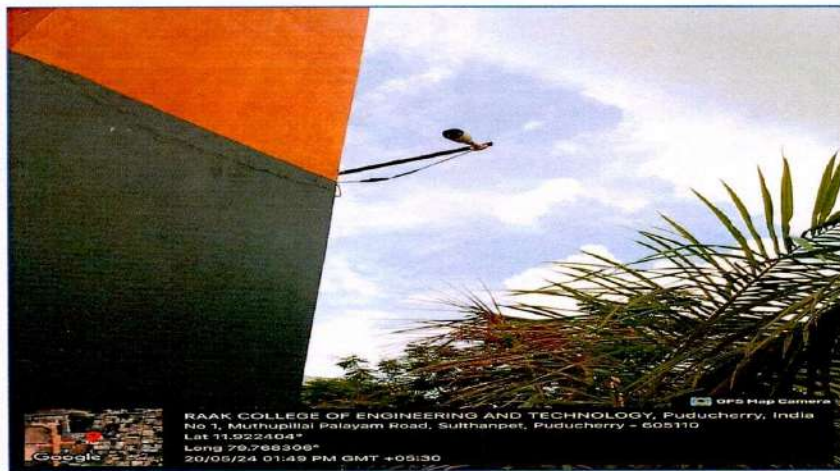
CCTV at the Entrance of Girls Hostel
