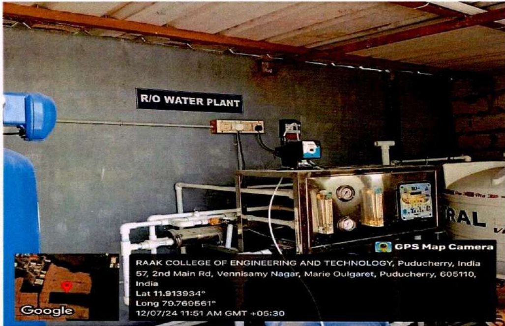
REVERSE OSMOSIS WATER PLANT
