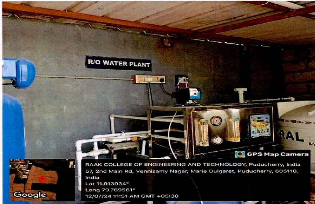
REVERSE OSMOSIS WATER PLANT
